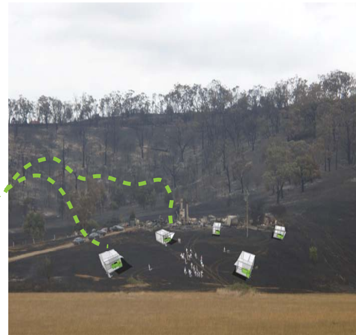
1 / pods delivered to site and then craned into position - providing immediate shelter, security and basic amenities.
